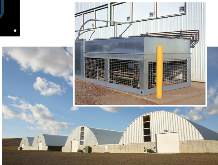
Storage Climate Controls
