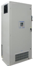
YASKAWA A1000 VFD to Chiller #1
