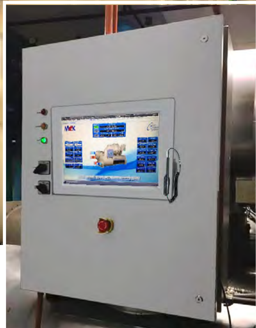
Industrial Control Panel Custom built by MCK using MCS Controls
