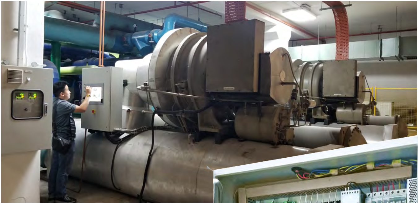
▲ MCK technician making final adjustment on MCS Touchscreen using MCS Connect
