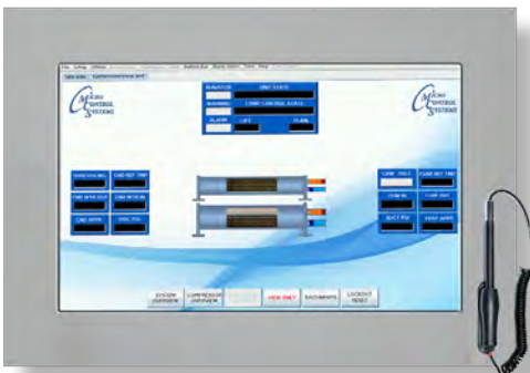
EVAPORATOR CONDENSER OVERVIEW SCREEN
