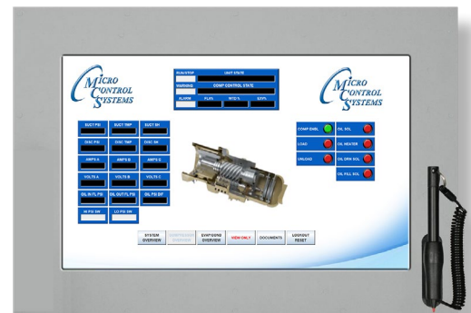
COMPRESSOR OVERVIEW SCREEN
