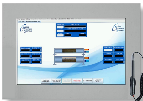
EVAPORATOR CONDENSER OVERVIEW SCREEN
