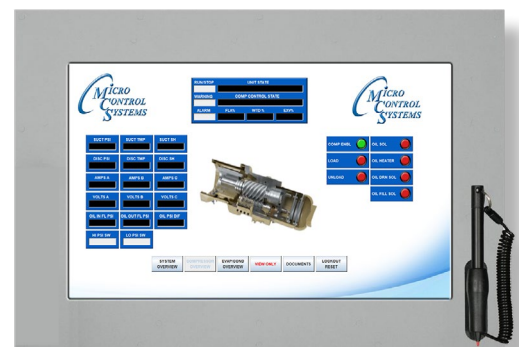
COMPRESSOR OVERVIEW SCREEN
