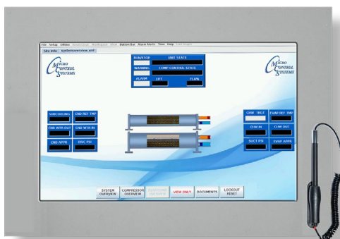
EVAPORATOR CONDENSER OVERVIEW SCREEN
