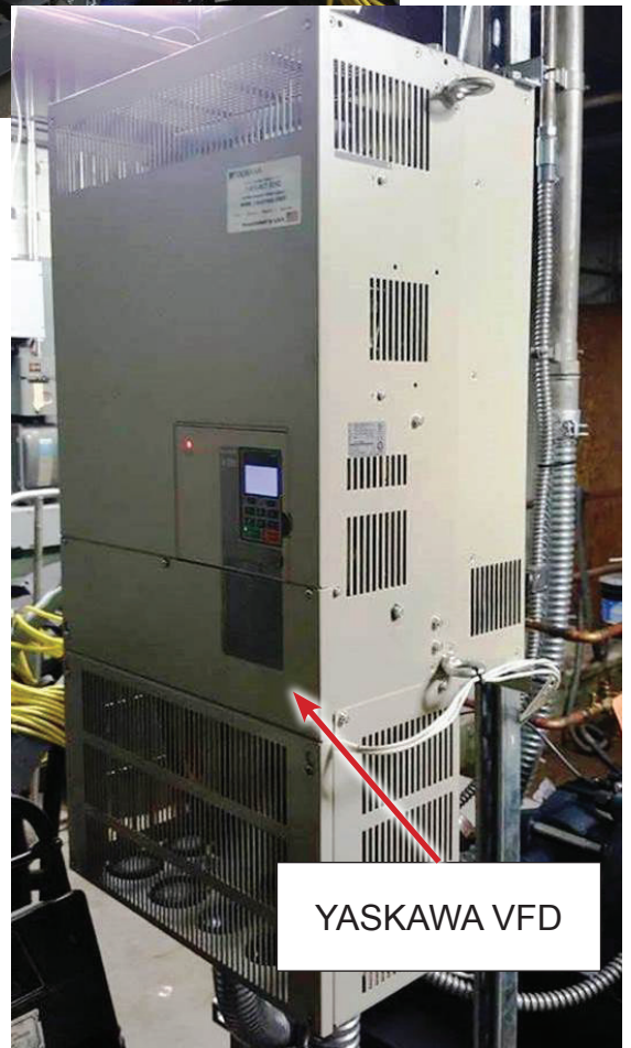
MCS CONTROL PANEL
