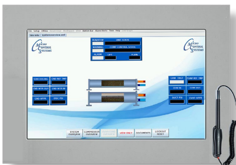
EVAPORATOR CONDENSER OVERVIEW SCREEN
